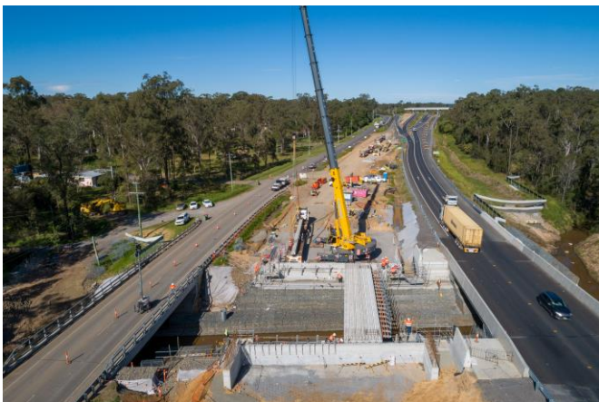
Image above: Installation of bridge girders to construct the southbound corridor Norris Creek bridge.
